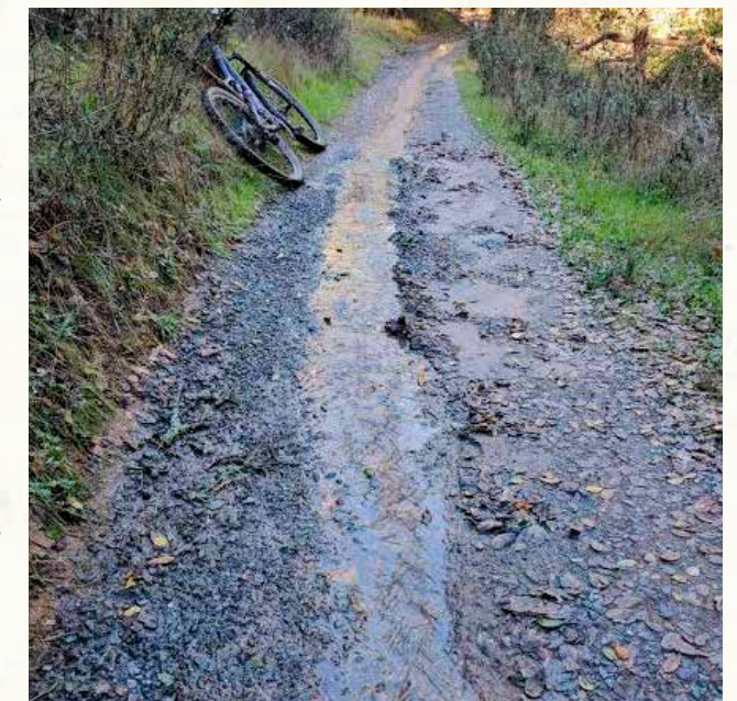
Result of insufficient grade reversal. Shoreline Trail, China Camp State Park
